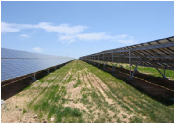
PV modules on the vast area
